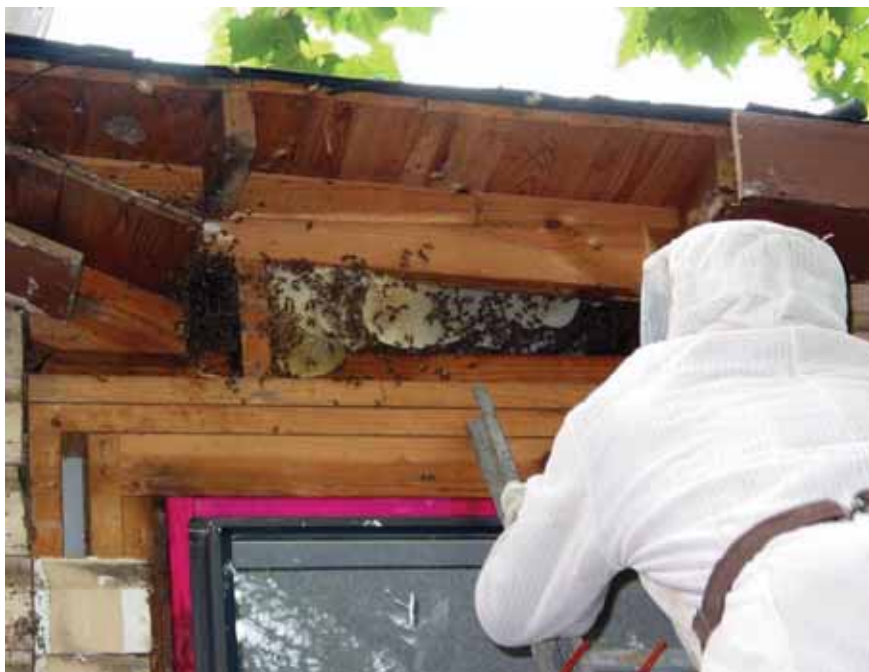
Figure 4. Honey bee nest and worker bees are exposed within a home wall void. Nest removal from buildings is a job for professional pest control services. Photo by Timothy Haley, USDA Forest Service, www.insectimages.org
