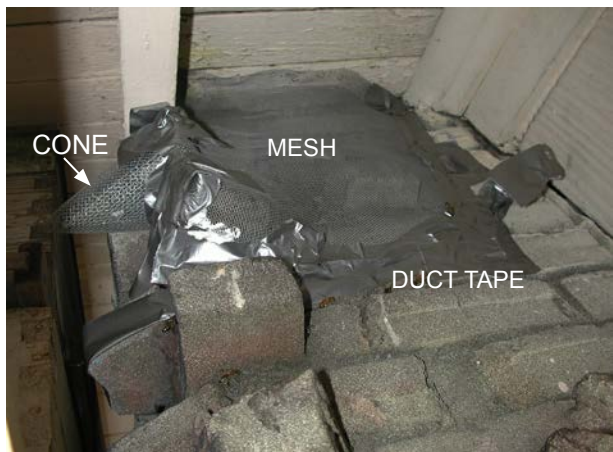
The escape cone and additional wire screening duct taped to chimney bricks.
